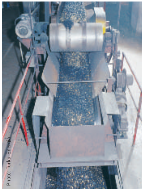
Pellets are mixed with coal before feeding into hammer mills
